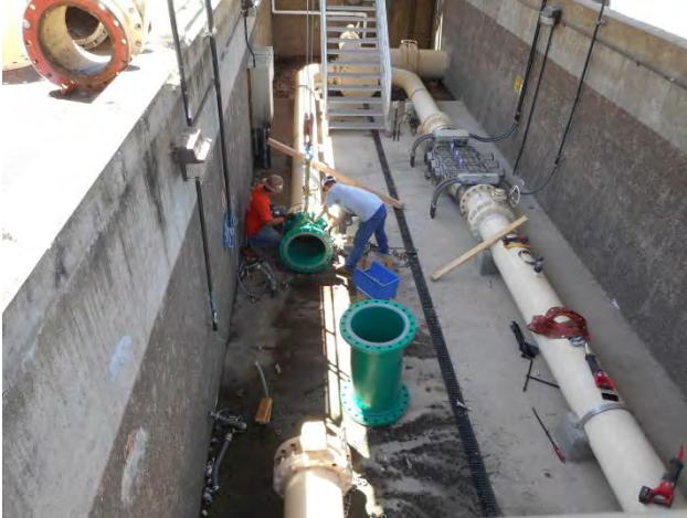
Stettler Supply has begun work on the replacement ultraviolet (UV) disinfection system
