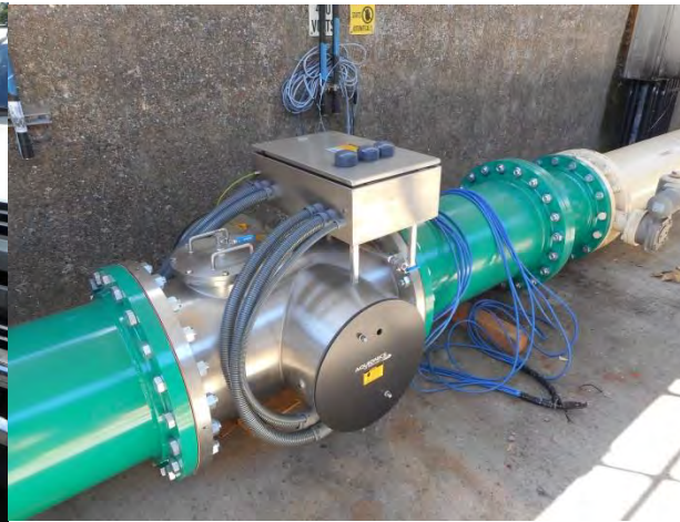
The new reactor chamber has been installed
