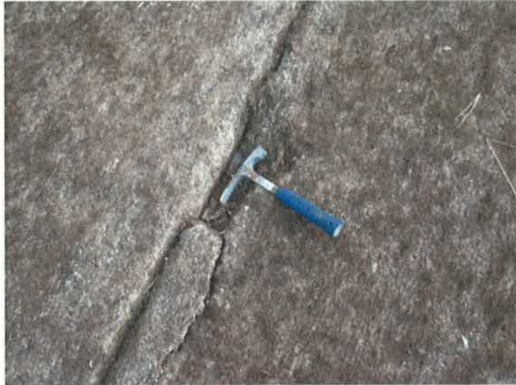
Concrete loss between spillway slabs
