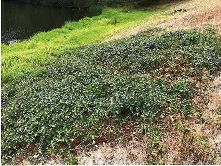
Vegetation growing on upstream embankment and near waterline
