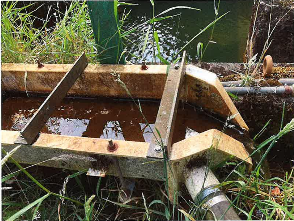
All the weirs were clean and functioning properly at the time of the inspection
