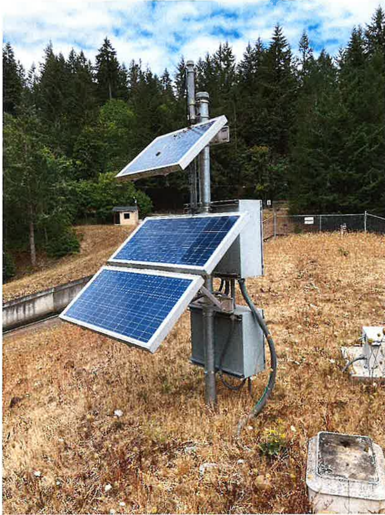
Monitoring station, clean and secured
