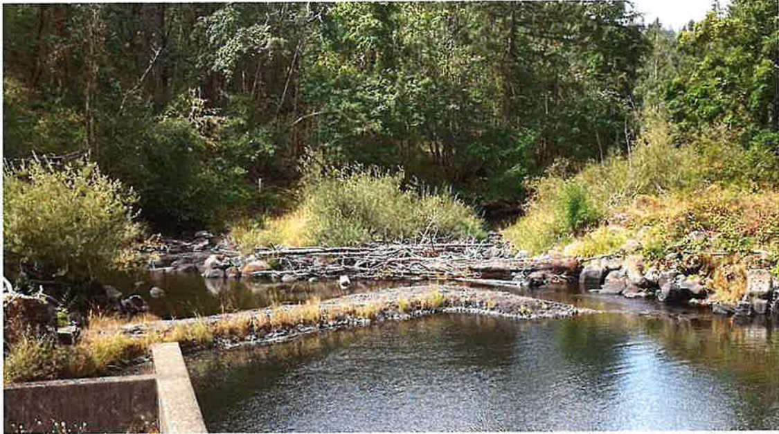
Logs on edge of discharge channel
